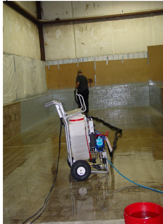
A polyurea coating is applied to a secondary containment area using the Graco Reactor® E-10.
